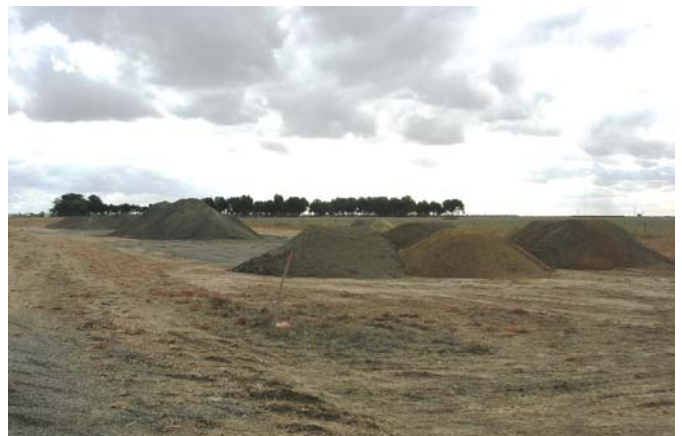
Stockpiling of soil and damage caused by roadworks on a native grassland roadside. Photo: DSE, Ballarat
